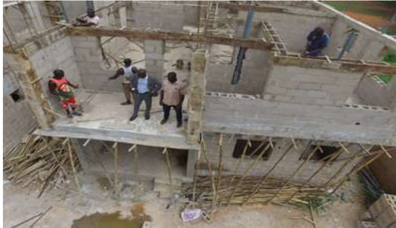
Figure 6. Workers in the upper floor were not wearing any Personal Protective captured by DJI drone. Source: Field survey 2019.
