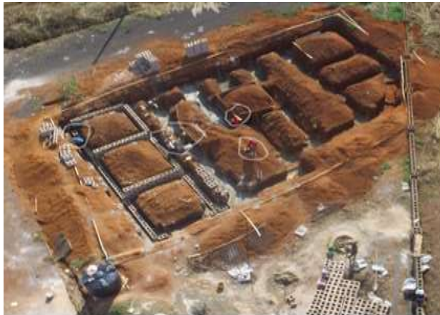
Figure 5. Worker in the foundation working without their personal protective equipment and the foundation basket dropped carelessly on the floor, captured by a DJI Phantom 3 Standard drone. Source: Field survey 2019.
